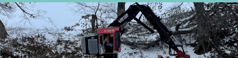
Clean up of large fallen trees at Cedar River Crossing.
